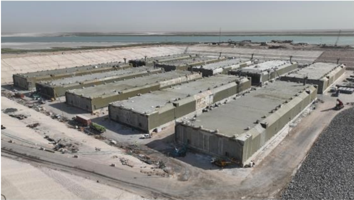
Figure 3: 10 Pieces of the Immersed Tunnel at the Work Site and Pouring Before Transporting Them.
