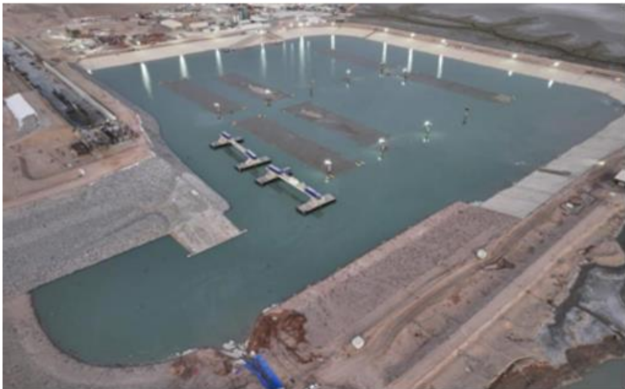
Figure 4: Submerging 10 immersed tunnel segments to apply Archimedes' principle in lifting the tunnel segments and preparing them for transport to the required location by sea.
